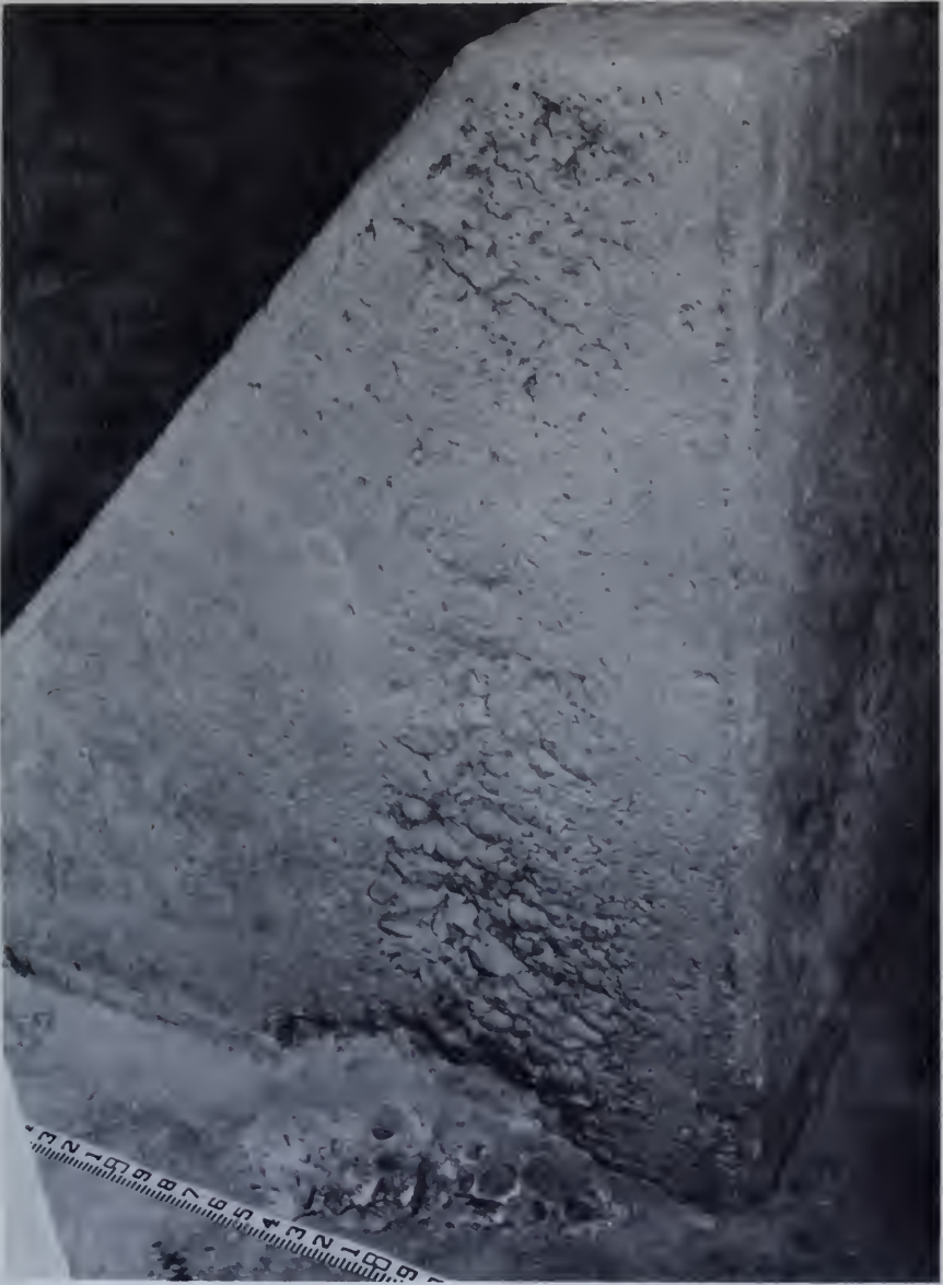
Figure 185. —A dentate in overflow weir stilling basin at Yellowtail Afterbay Dam showing typical cavitation damage. P459-D-75010.
